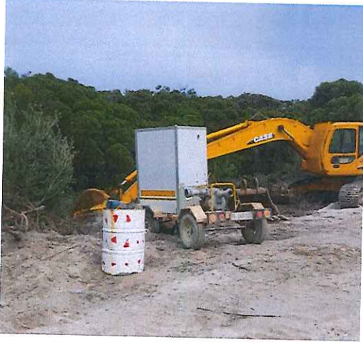
Figure 15: Ablution facilities and refuse bin.
